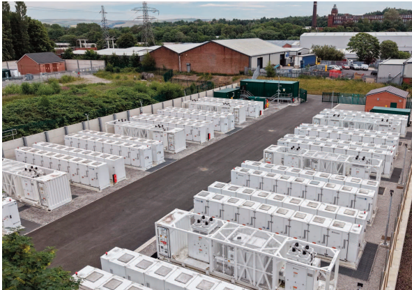
Beyond battery storage, Masdar is a leading investor, developer, and operator in the UK offshore wind sector —WAM
