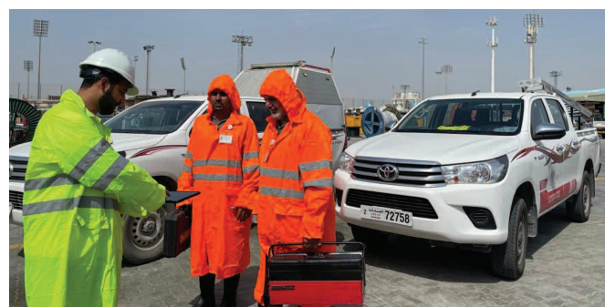
Sharjah Electricity, Water and Gas Authority conducted repair and maintenance operations in the central region, alongside electrical stations and transformers across all areas, to address the electrical faults resulting from the exceptional weather conditions. —WAM
