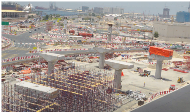
Al Shindagha Corridor Improvement Project included a two-lane tunnel extending 500 metres for left-turn traffic coming from Khalid bin Al Waleed Road heading to Al Mina Street with a capacity of 3,200 vehicles per hour —WAM
