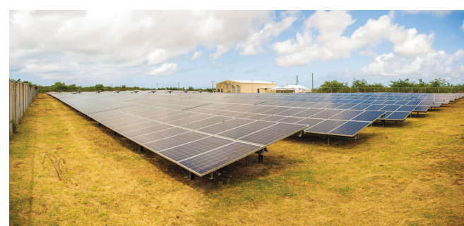
Khazna PV project will involve the development, financing, construction, operation, maintenance, and ownership of the plant and associated infrastructure —WAM
